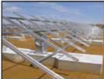
SOLAR MOUNTING SYSTEM
