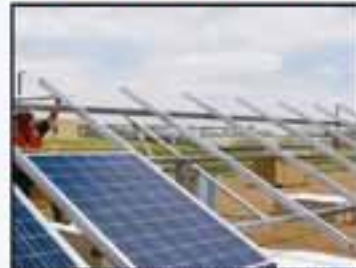
SOLAR MOUNTING SYSTEM
